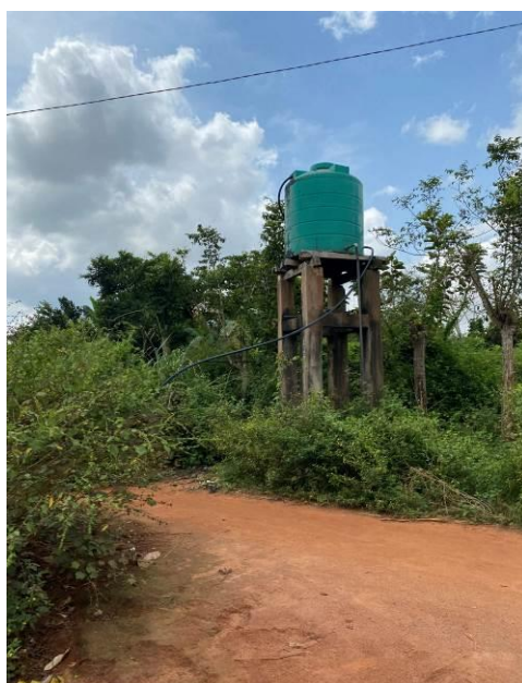
Figure 5.26: Example of water facility in one of the villages of the Aol
